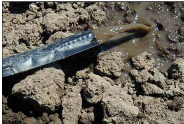
Figure 12. Dirty flush water. This is an indication of impending plugging problems
